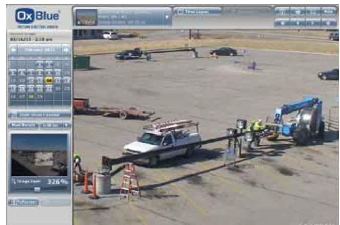
OxBlue construction cameras monitor the installation of solar panels at a Walmart and OmniWind turbines in a parking lot — both short projects that require close monitoring.
