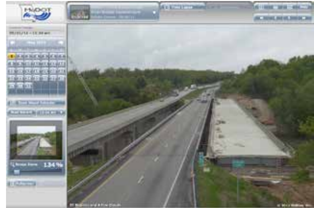
Rather than tie up traffic for weeks by building the new bridge piece by piece at the site of the existing bridge, the general contractor built the new bridge next to the old bridge.
