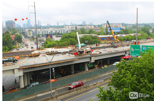
Image taken from OxBlue’s fixed-position camera located at the I-85 construction site.
