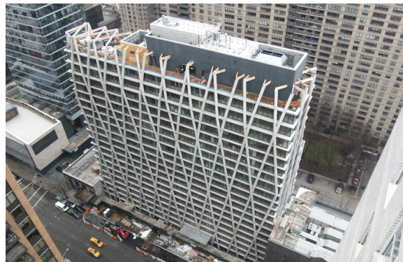
The OxBlue construction camera monitoring Equity Residential's 20-story, 236-unit building on Manhattan's Upper West Side enhances project transparency and insight for the developer.
